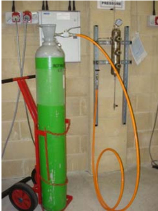
Figure 10, cylinder connected to charging equipment
