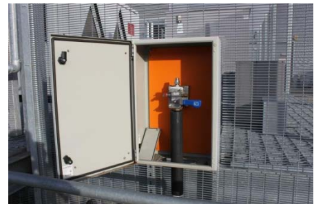
Figure 14, example of a remote charging point
