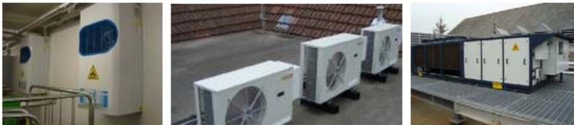
examples of equipment designed to contain hydrocarbon
